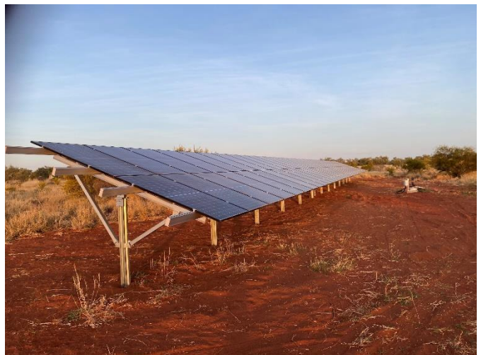
The newly installed production bore and solar array
